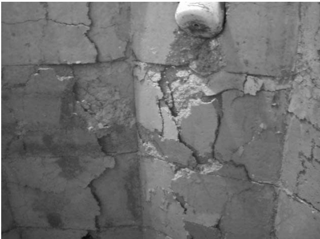
Picture 4 Cooling stripes area: the damaged refractory below an oxygen lance
